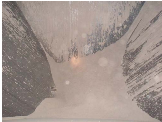
Figure 2: Dust Bridge in Hopper
